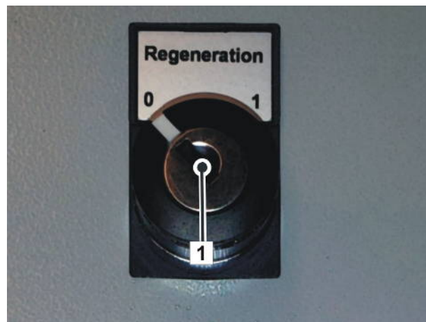
Fig. 12; the "Regeneration" key-operated switch
